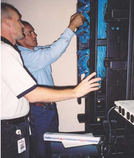
Barron Rascoe (L) and John Murphy (R) review the structured cabling installation in progress.
